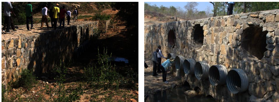
Fig 6: A nearly complete Rwemhepo Bridge in ward 5, Image source: ECLF (picture taken 12 May 2017)
