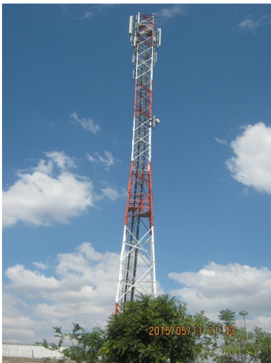
Figure 2.14 35m Mobile tower base station at St Georges in Emerald Hill area, near The Chase Note: All bands available as evidenced by presence of dual band antennas at top (900 +1800Mhz) and 2100 (3G) at the bottom on single band antennas].
